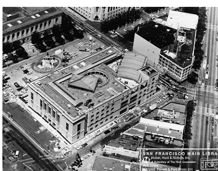
Aerial view at construction of new Main Library exterior, June 5, 1995. Image courtesy of San Francisco History Center
